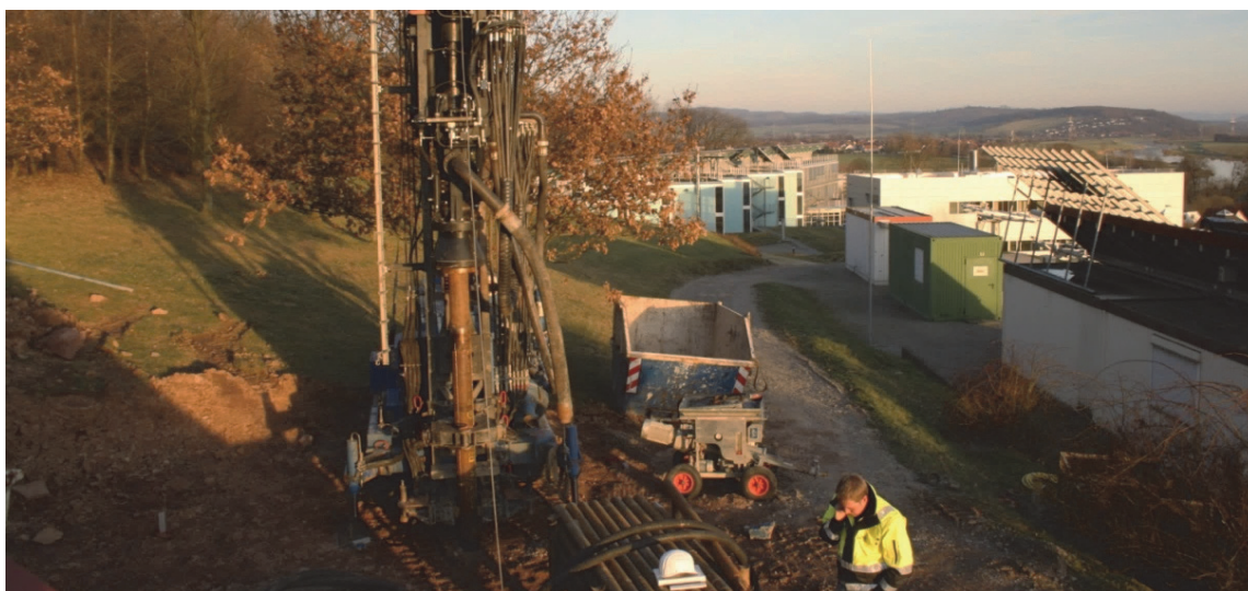
Figure 2-6: Drilling of a borehole for a vertical ground heat exchanger at the experimental ground heat exchanger field at ISFH, Emmenthal
