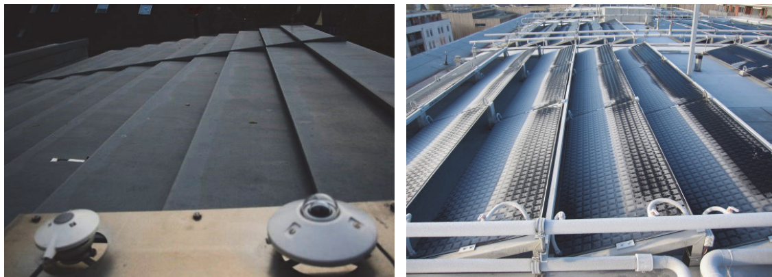
Figure 2-19 Uncovered collectors: Left metal roof collector in operation with condensation on the roof elements (darker grey). Right: Selective uncovered collectors with hoarfrost in the morning partly melted by sunlight [source Energie Solaire SA, Bernard Thiessen]
