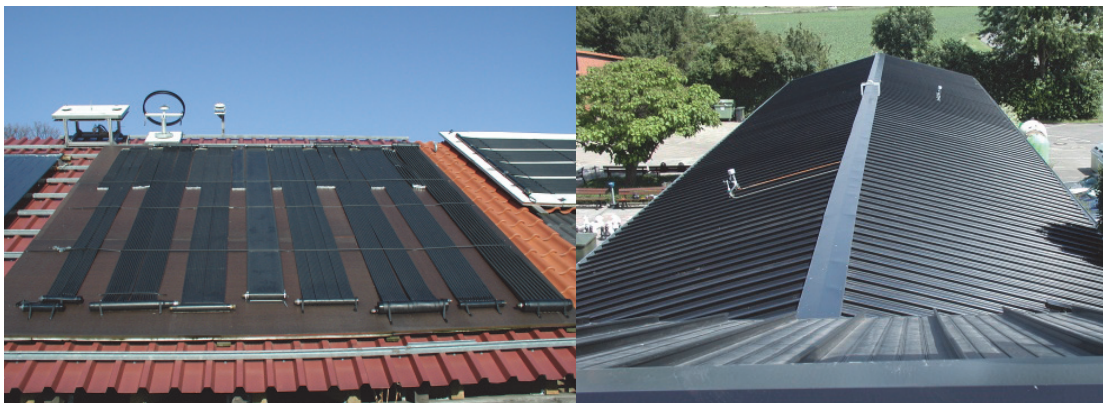
Figure 2-17 Uncovered collectors: Left 8 different black polymer collectors during testing at ISFH, right: 650 m 2 of black metal roof collector for swimming pool heating in Nordstemmen, Germany
