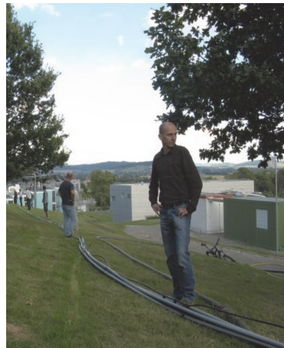
Figure 2-9: An approximate line source: 70 m of double U-tube ground heat exchanger just before inserting it into a borehole
