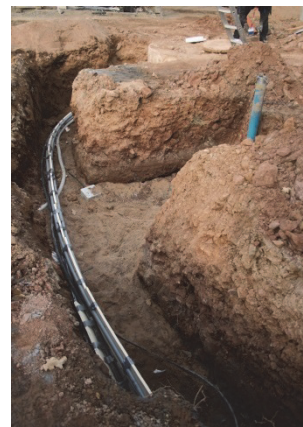
Figure 5-22: Buried horizontal connecting pipe at ISFH test facility
