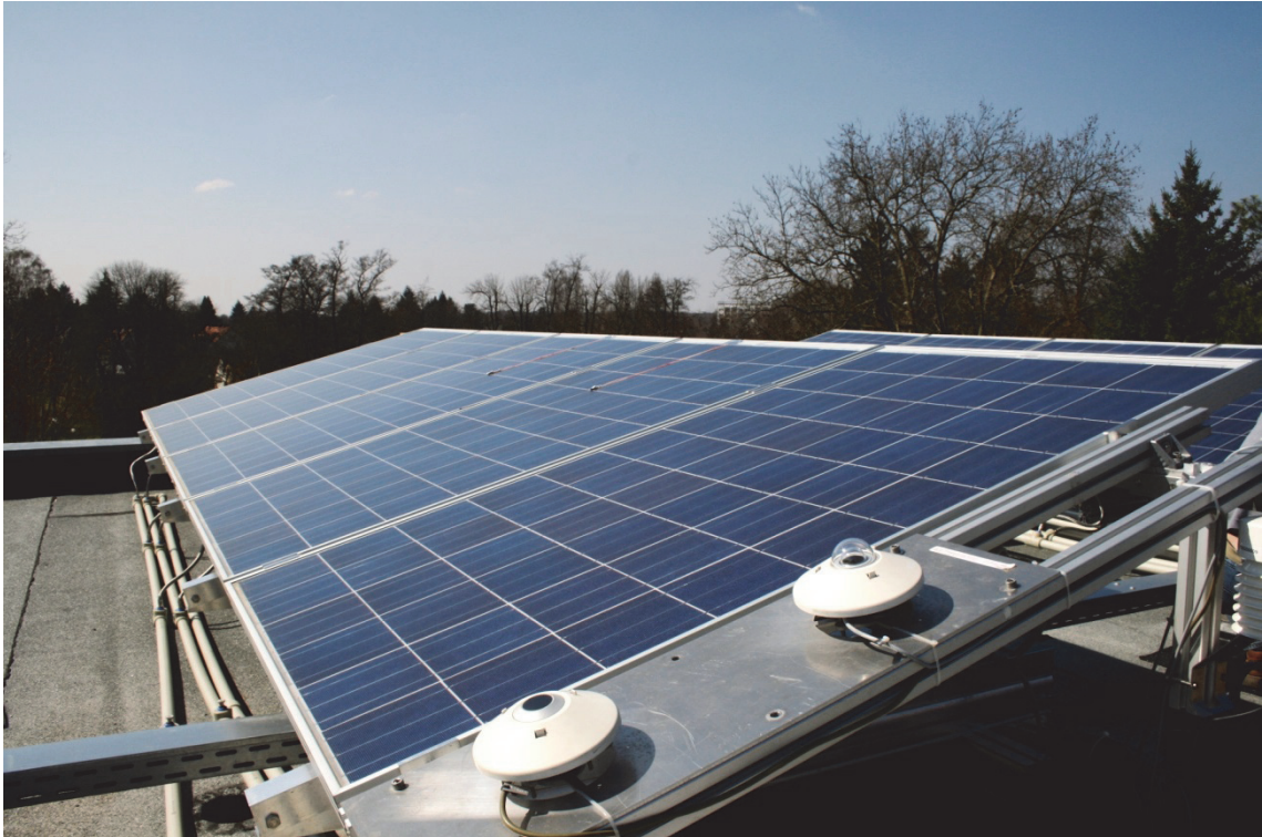
Figure 6-2 System in Dreieich with PVT- collectors; front: Meteorological weather unit with pyrgometer and pyranometer
