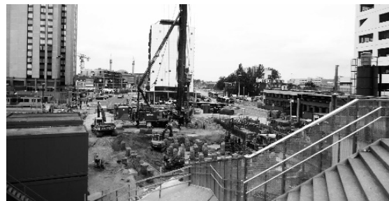
Figure 104 Construction of the WTC building in front of the city hall. Source: aurora, 2016, 2017 respectively.
