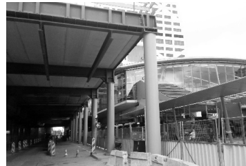
Figure 64 Small elevated square of immediate access to the west sector station and future enlargement - Forum (under construction); Source: author, 2017.
