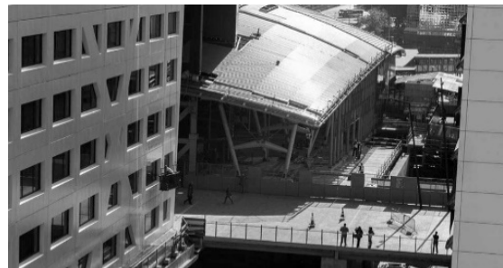
Figure 103 Station, at the time under construction, no current staircase and old connecting catwalk between the banks. And aerial view of the transformations in progress on the west side. Source: CU2030, 2016.
