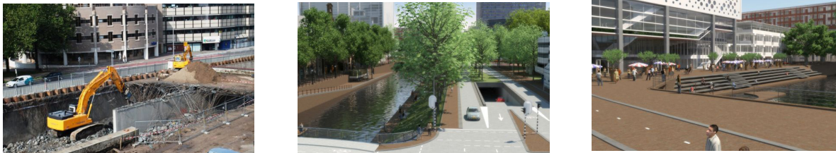
Figure 45 Demolition of the avenue and design of the Catharijne Channel north sector already built. Source: CU2030, 2017.
